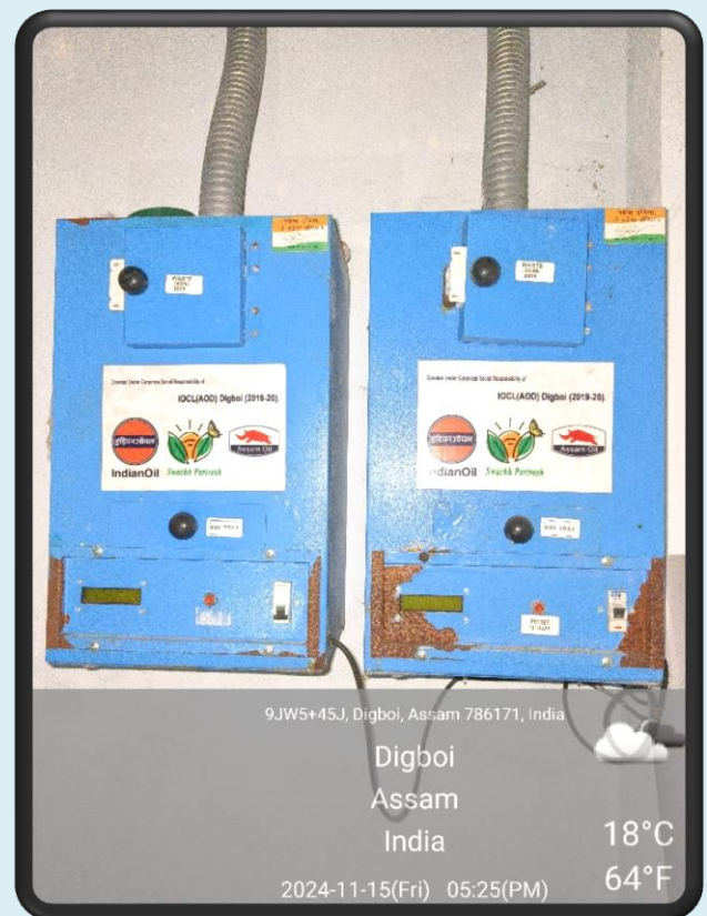
Sanitary Pad Incinerator of Girls' Common room
